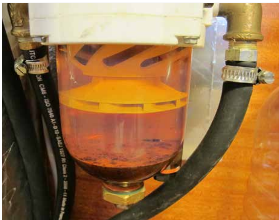
Fuel in a primary filter should be absolutely crystal clear (although colors may differ according to diesel blends and added dyes). Any opaqueness is a sign of serious contamination that needs addressing.
